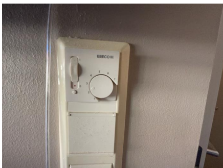
Termostatbryter for varmekabler.
