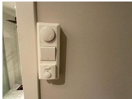
Termostatbryter for varmekabler.
