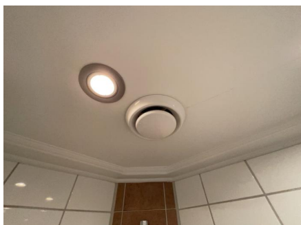
Lufteventil i himling.
