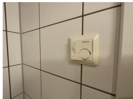
Termostatbryter for varmekabler.
