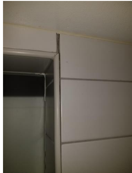
Overflater vegger - [Riss flisfug bad]
