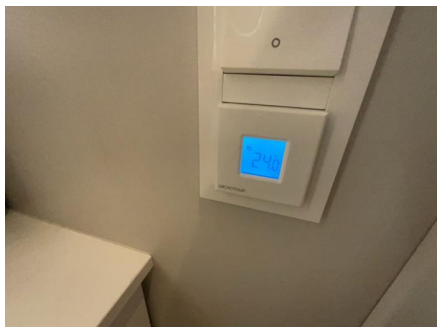
Termostatbryter for varmekabler.
