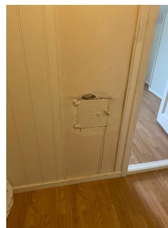
Manglende plate under feieluke (eldre type).
